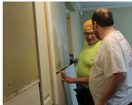
Jim Meis (Christ, Cedar Rapids) and Brad Gipple (All Saints, Indianola) installing drywall. Photo credit: Meg Wagner
