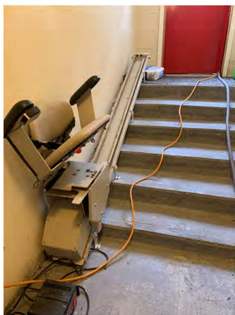
Old, broken stairlift
