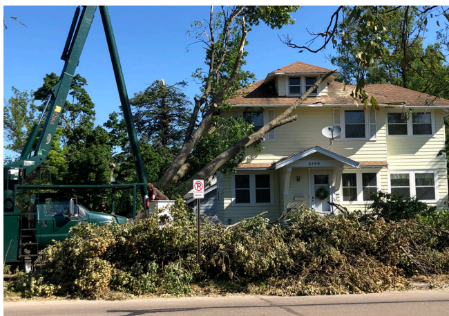
A crane is used to help remove a tree from a home in Cedar Rapids. Photos: Lauren Lyon
